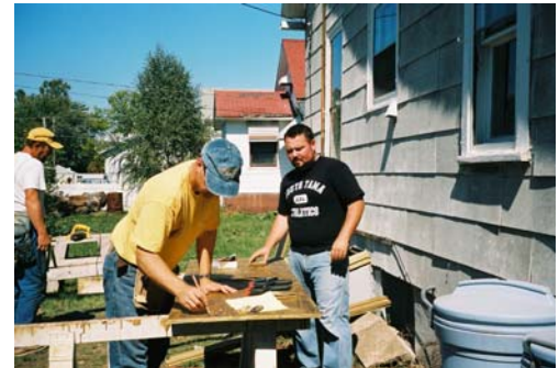
Volunteers install a new cellar door, adding safety and accessibility to the home of some Rock Island seniors.
